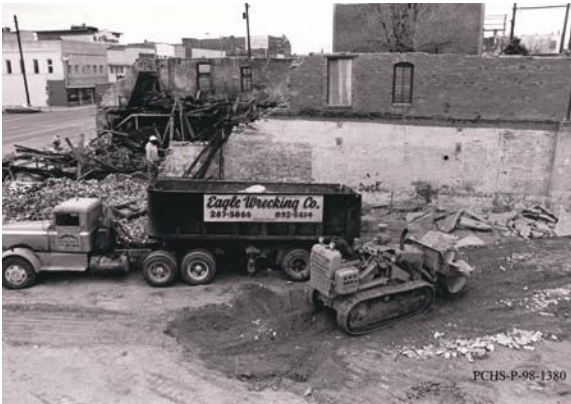
Figure 1.13. Excavation work was one of the first tasks in the construction of the Sangre de Cristo Arts Center, a long-anticipated addition to downtown Pueblo. (photo courtesy of Pueblo County Historical Society, PCHS-P-98-1380, John Suhay Collection)
